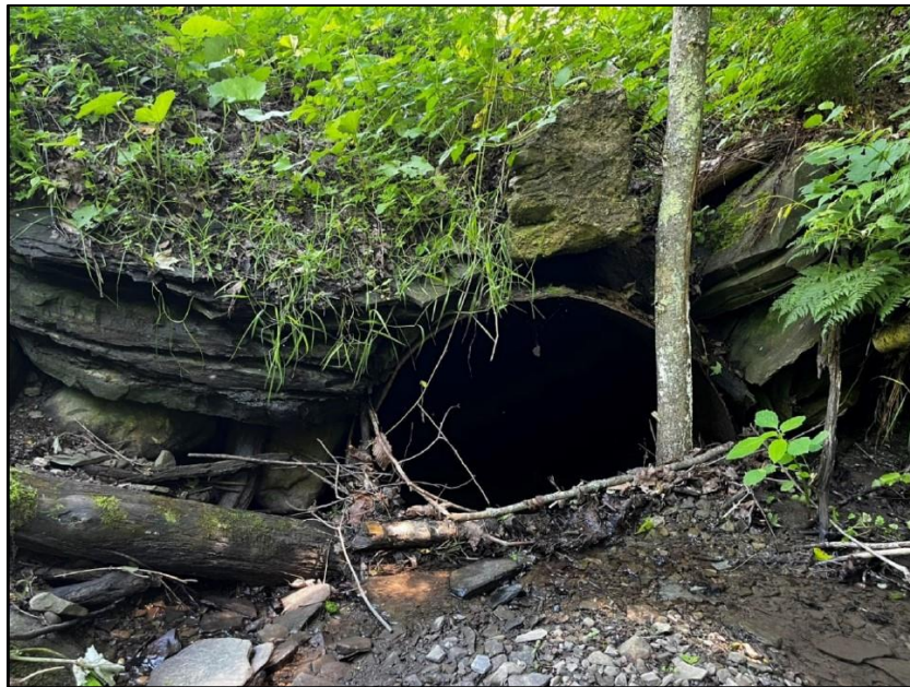
Pictured above is a photo of the Wright Road culvert inlet showing trapped debris and sediment. Photo by EcoStrategies Engineering & Surveying.
