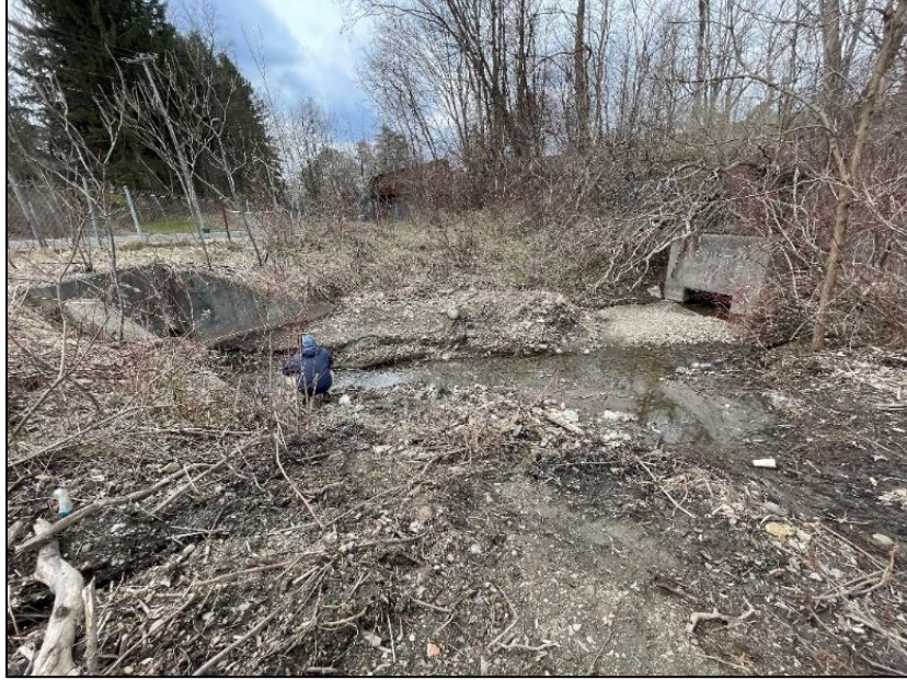
Pictured above is a view of the Fairmount Avenue site looking west from the east side of basin. Note excess sediment accumulation on western side of basin near main flow channel.
