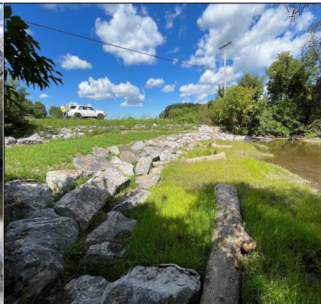
Pictured above is the Stow Road Bend after substantial completion, including a bendway weir pictured at the bottom right of frame.
