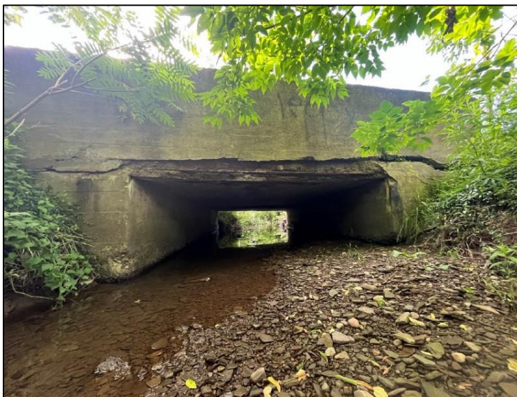
Pictured above is a photo of the Elmwood culvert outlet showing deteriorated concrete with spalling, cracking and exposed rebar. Photo by EcoStrategies Engineering & Surveying.
