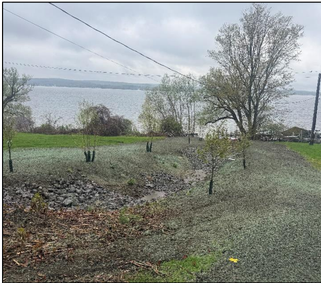
Photo of final plantings and grass-seeding work can be seen at Floral Avenue (Photo by Town Highway Department).
