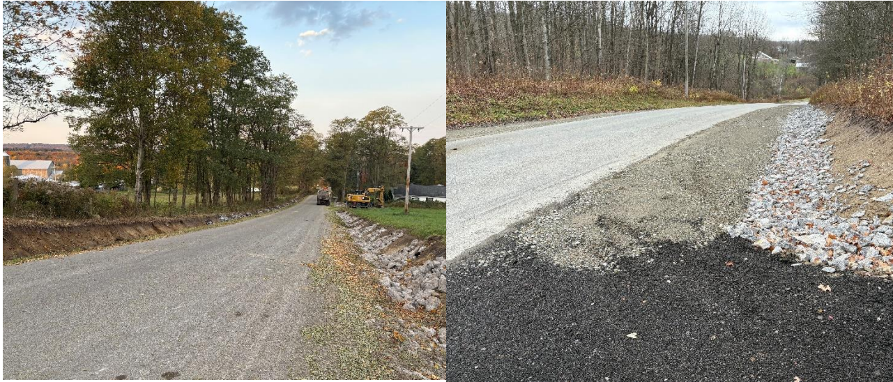
Above: Swale construction can be seen along Haight road, left, and Burdick road, right.
