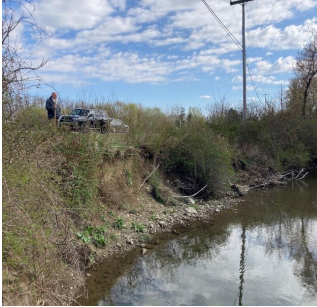
Pictured above is the Stow Road bend of Ball Creek prior to construction.
