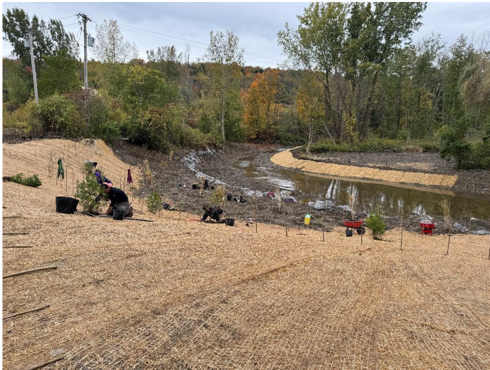
Figure 1. Pictured above, workers install native plantings along the Phase 2 stream stabilization of Ball Creek in the Town of North Harmony.
