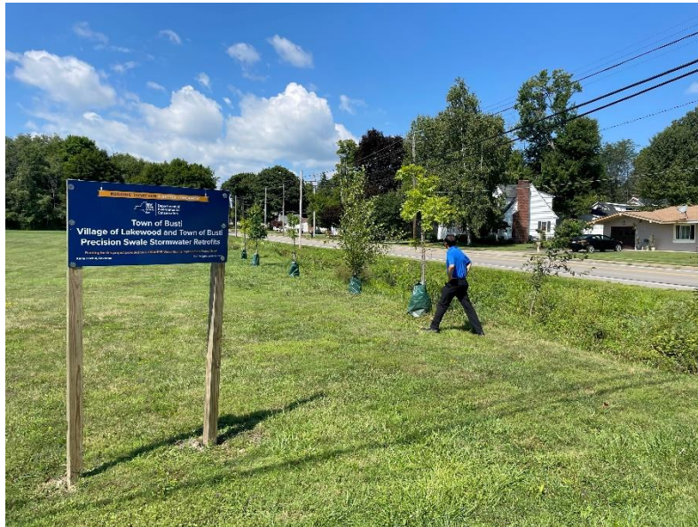
Figure 1. The Town of Busti's swales stabilization project, seen above along Summit Avenue in Lakewood, includes stormwater management work designed to reduce the causes of harmful algal blooms in Chautauqua Lake.
